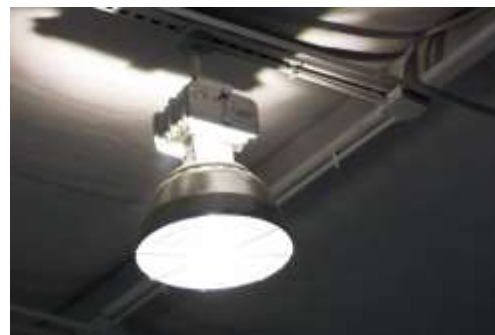
Figure 2. Mercury Vapor Lamps
